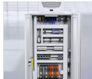
The electronic control devices, safety engineering and industrial PC are installed in the control cabinet .
