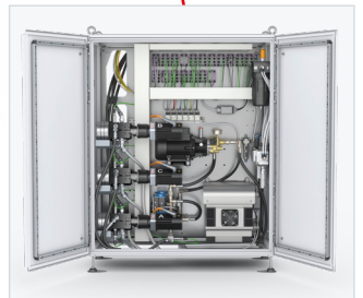
The dosing machine cabinet contains the components of the dosing periphery, e.g. the dosing pumps.
